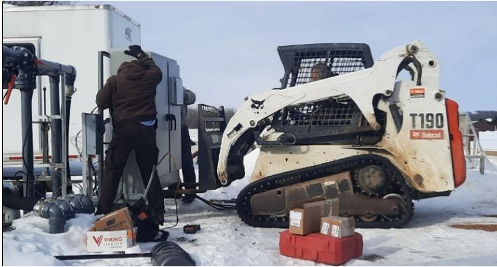
Zach and Jeff work with an electrician to install the new electrical panel at the pump station. Photos: Beth Glidewell/USFWS.
